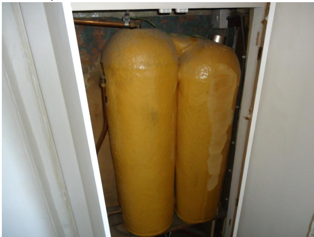
Hot water cylinder
