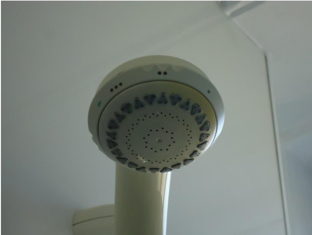
Shower room shower head (electric shower)
