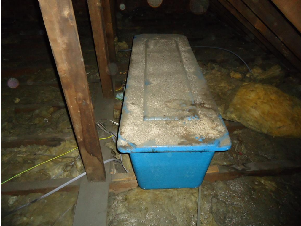
Cold water tank
